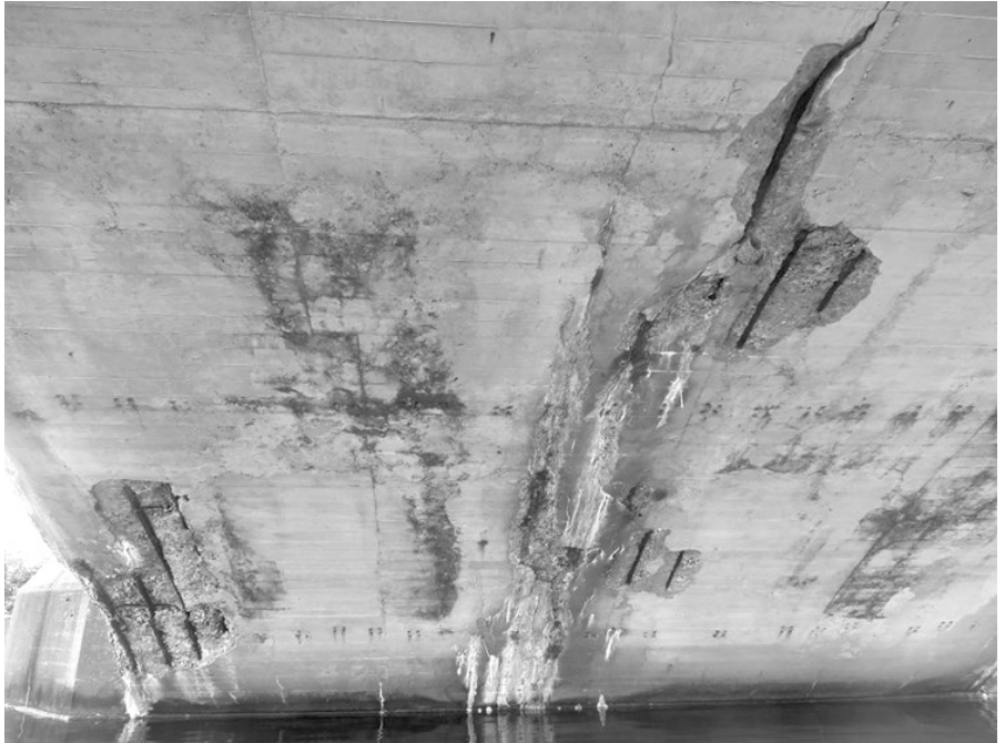
The use of deicing chemicals like salt has resulted in corrosion of some of the steel reinforcing within the concrete arches. Photo: Ohio Department of Transportation
