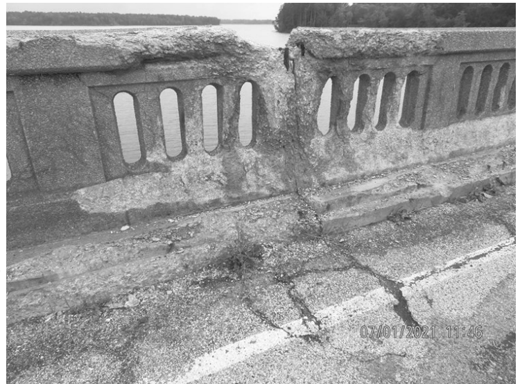
The open concrete railings on the bridge have deteriorated as salty snow was piled against them over the years. Photo: Ohio Department of Transportation.
