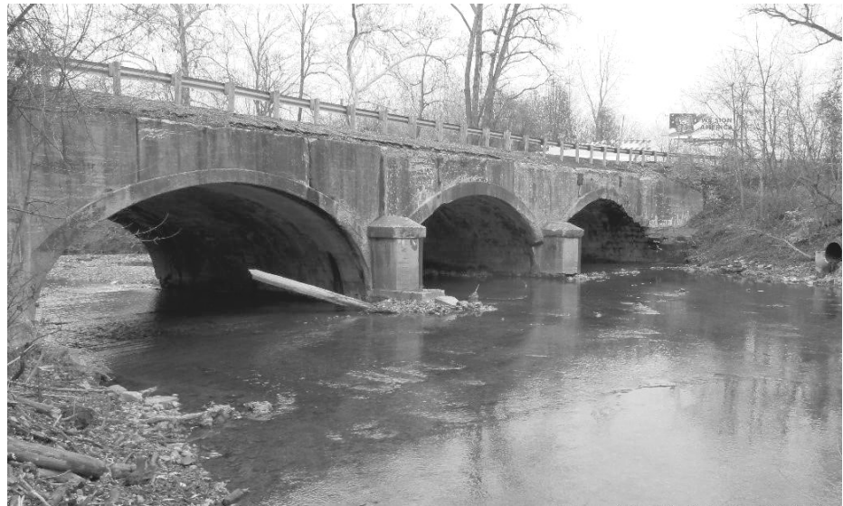
From the side, the Cherry Valley Road Bridge appears to be a run-of-the mill concrete arch bridge. Photo courtesy Rod Lemasters
