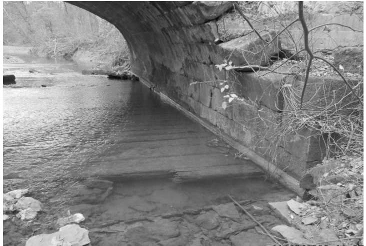
A close look at the interior of the arches reveals their original canal design of cut stone laid up on a wooden cribbing and platform in 1835.
