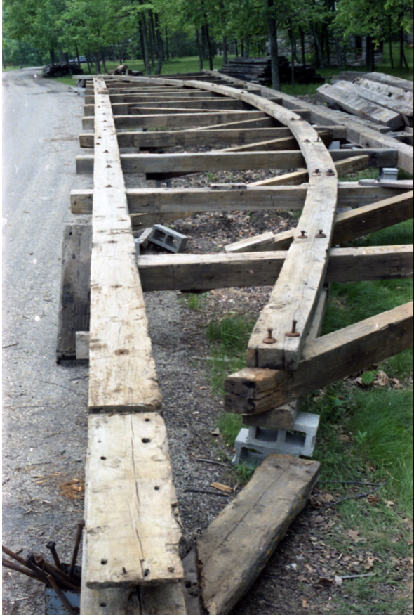
← A contractor was still assembling the relocated trusses at the new location in Bebb Park when Diehl visited in May 1968.
